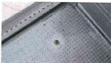
Drain in the floor pan.
